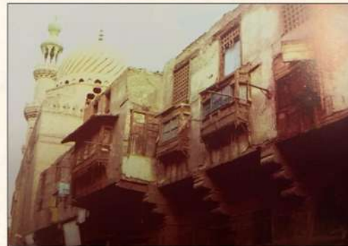
Rabbe Al manistrili before dilapidated 1993
